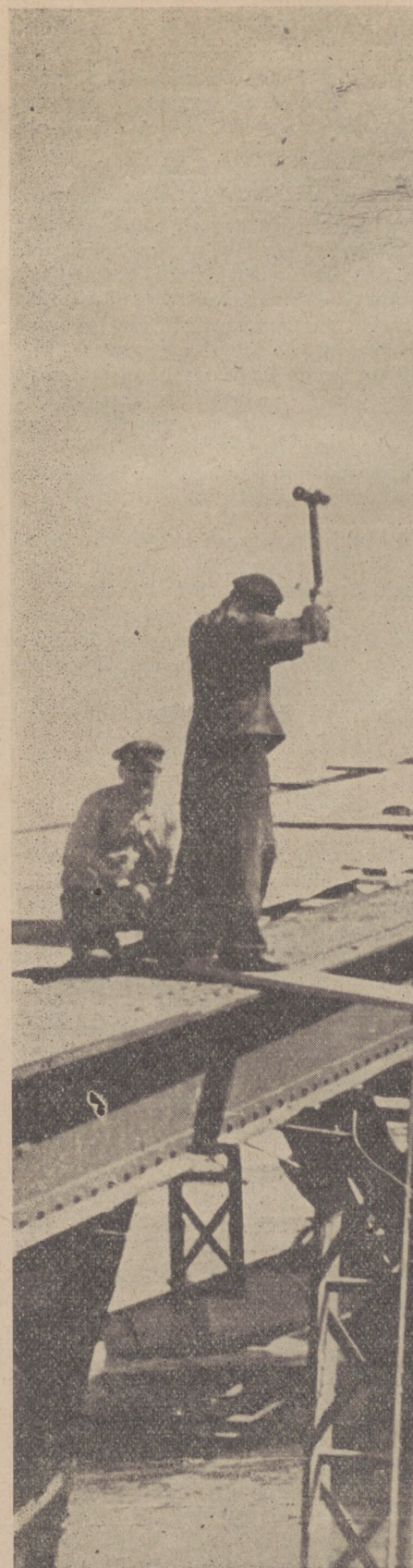
"EVERYONE WAS WORKING FOR RECOVERY..." These men are rebuilding one of Warsaw's railway bridges.
