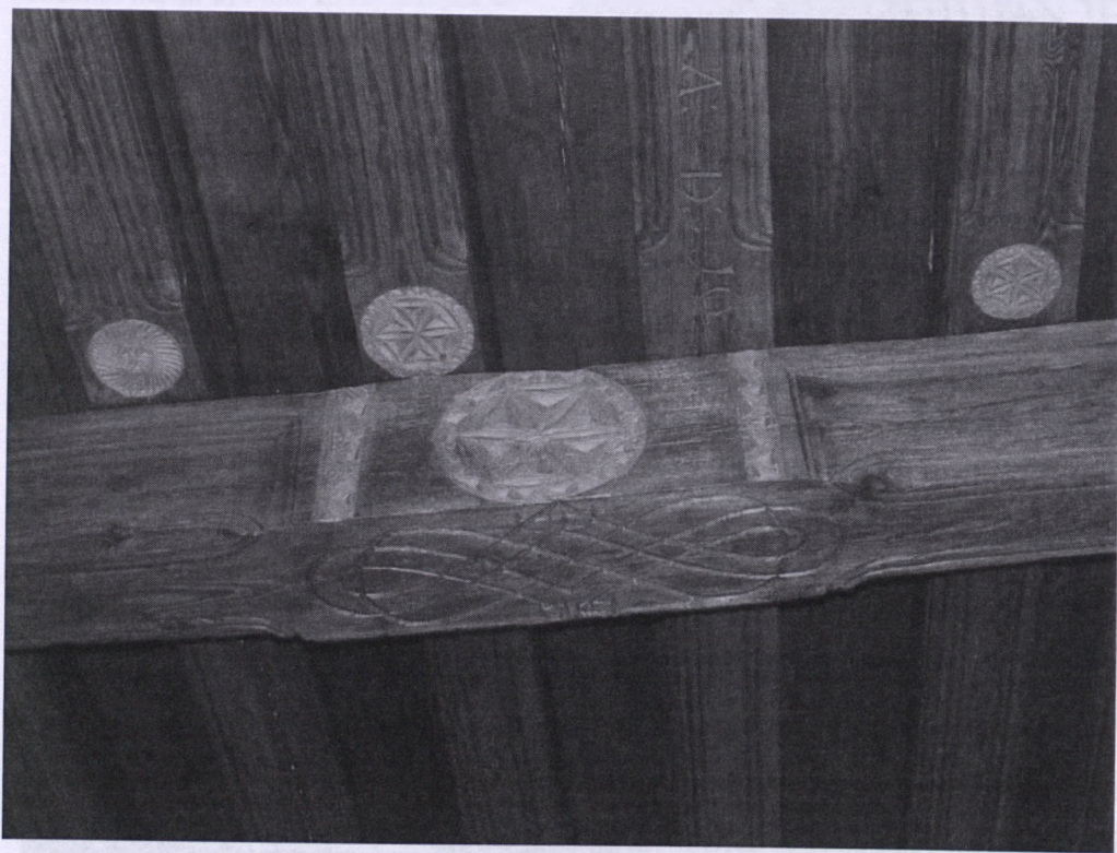
Fig. 2. Large rosettes situated on vertical walls of the cross-beam and adjacent beams. The interior of the tenement house on Ormiańska 26 Street
