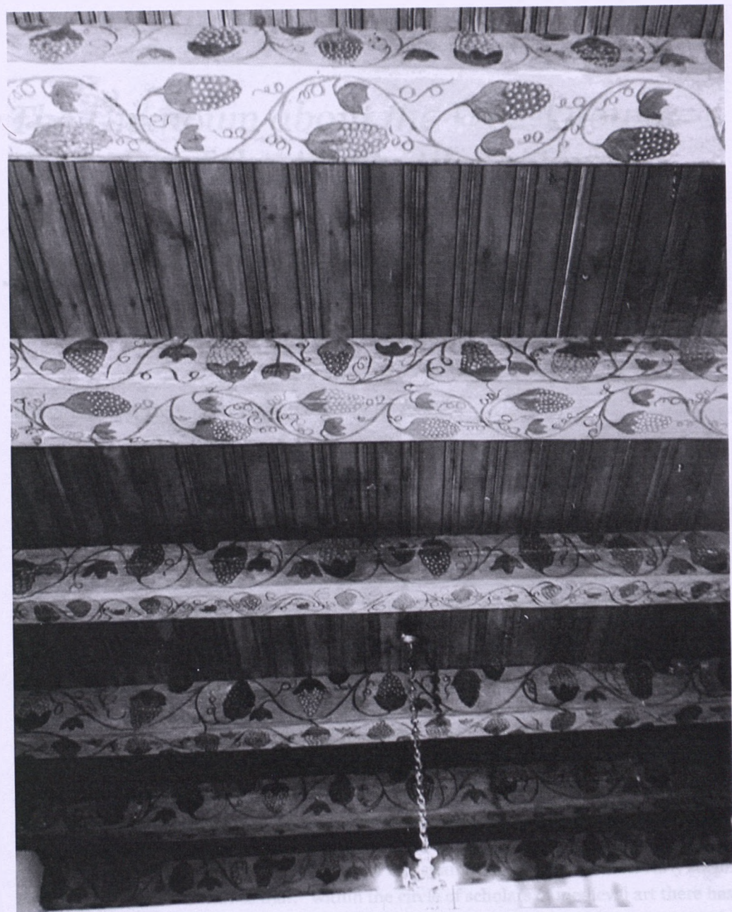
Fig. 13. Ceiling beams decorated with a motif of floral flagella. The interior of the tenement house on Staszica 29 Street
