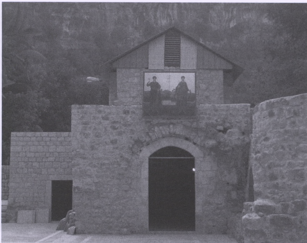
Fig. 7. Church in Kaftûn with a new roof protecting the murals in the upper parts, photo taken by M. Łaptaś
