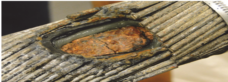
Fig. 6a. The return cable damaged on the Swedish – Polish Link, image 1 [own source]
